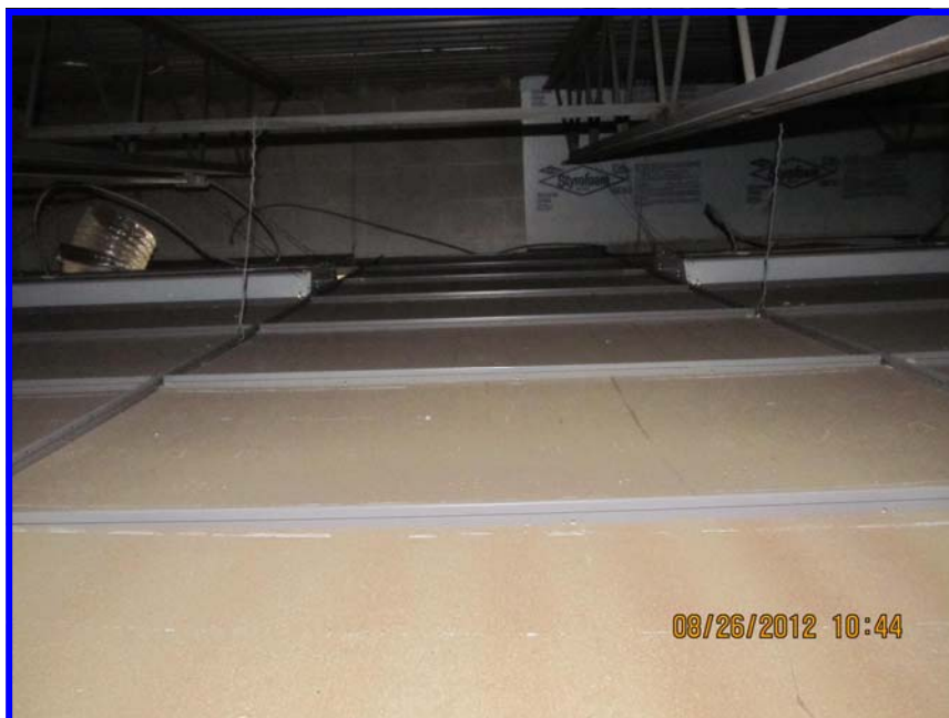
ROOM # 1-CEILING TILE ABOVE TILE-AFTER CLEANING
