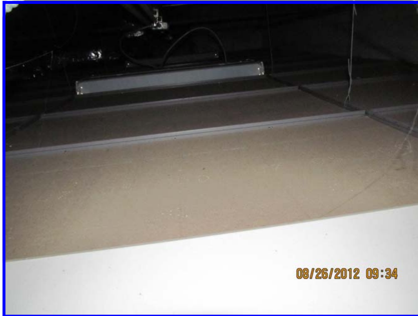
ROOM # 1-CEILING TILE ABOVE TILE-AFTER CLEANING
