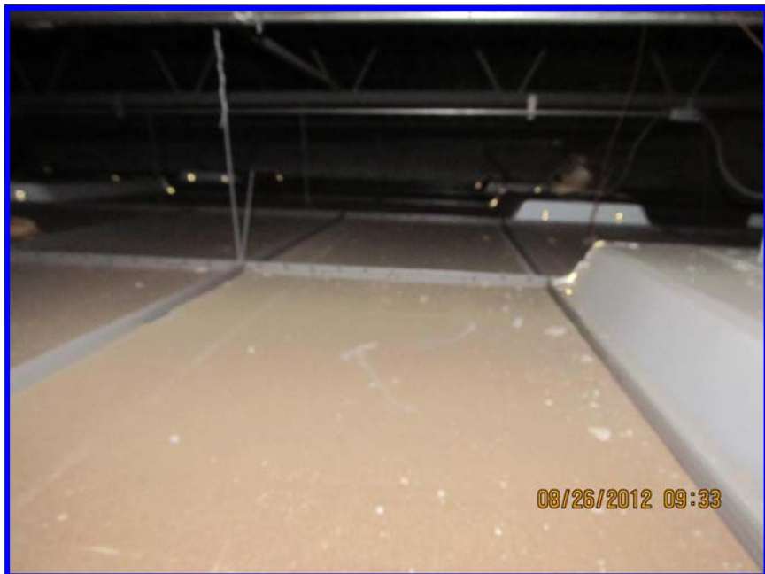
ROOM # 1-CEILING TILE ABOVE TILE-AFTER CLEANING
